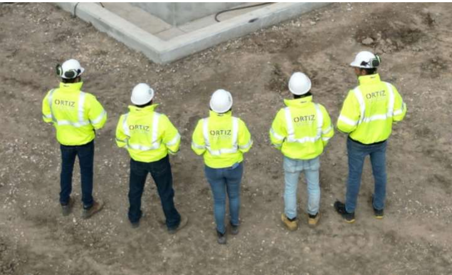
Energy specialists in Grupo Ortiz. Photovoltaic energy, 7V Solar Ranch Project. United States
