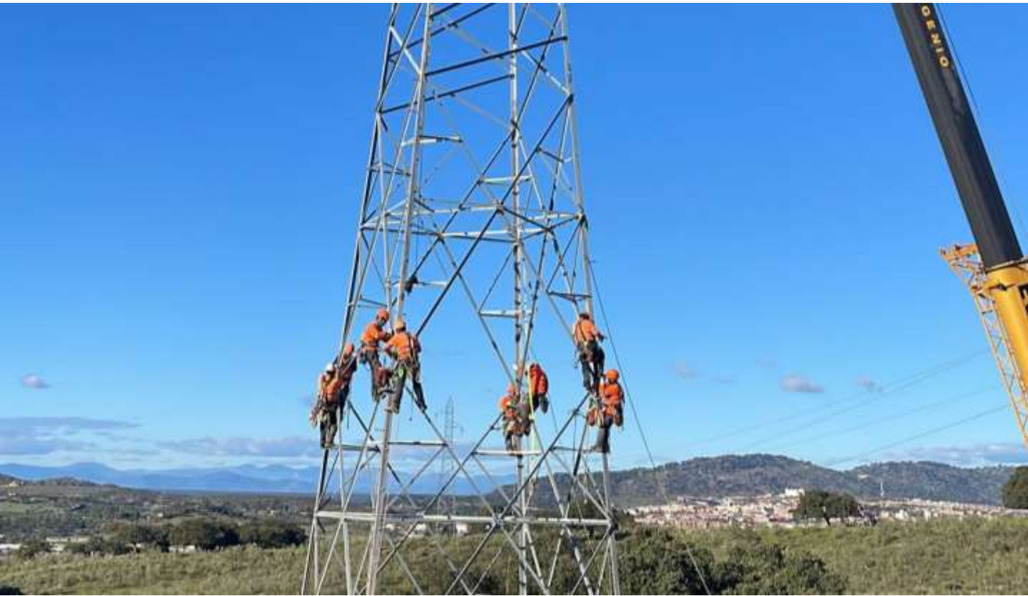
Infrastructure for the evacuation of power from renewable farms (wind and photovoltaic). Spain 2022
